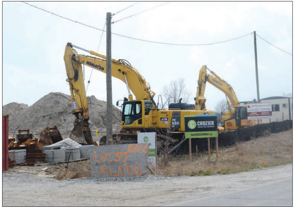
MAKING PROGRESS – Flato Development's plan for Phase 2 of their Beeton development has been ratified by the Town of New Tecumseth. Phase 1 of the development, located on the south side of Main Street, beside the cemetery, is already underway. BRIAN LOCKHART PHOTO
